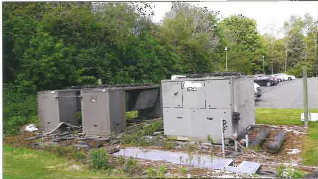
Fig 4: Redundant plant (location of proposed additional parking)
