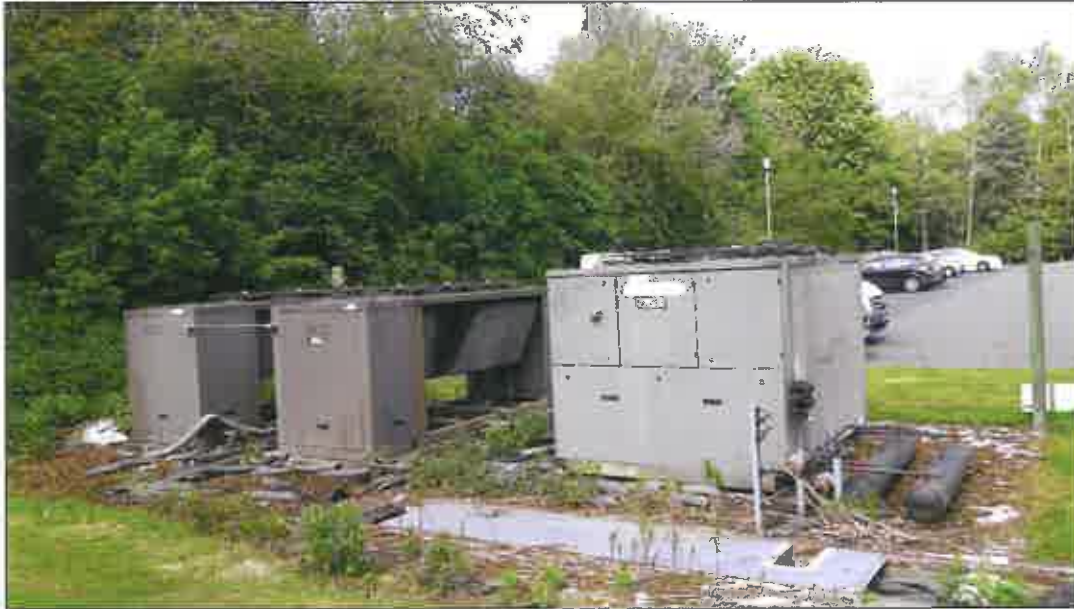
Fig 4: Redundant plant (location of proposed additional parking)
